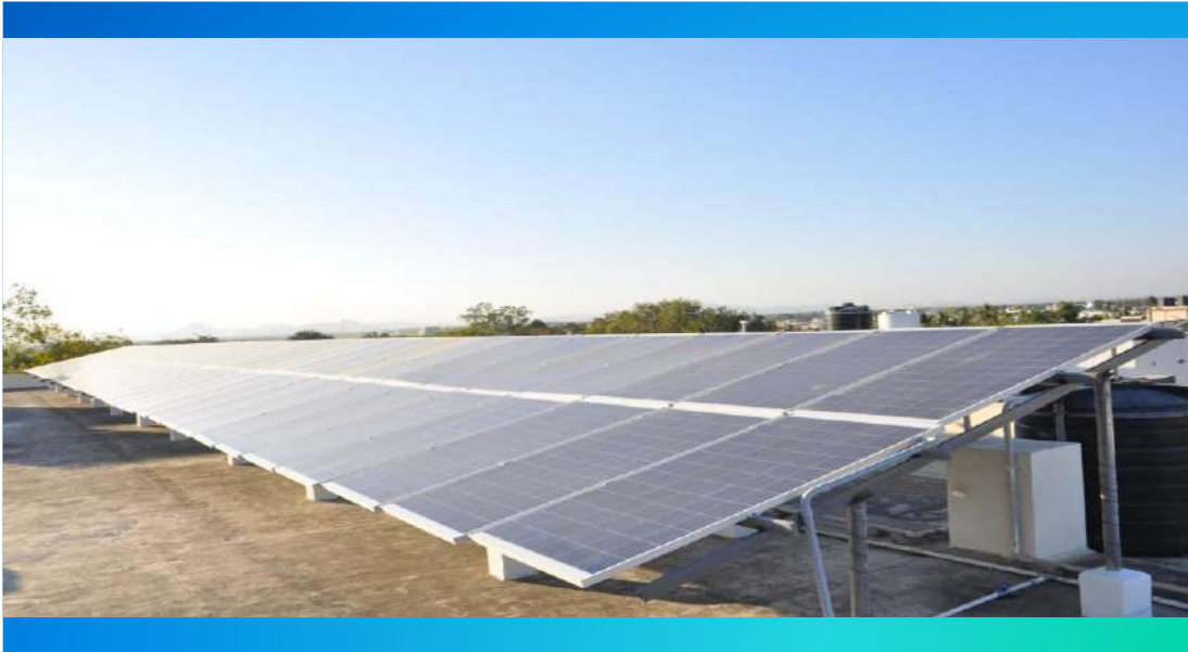
Solar Panels installed in John Med Block
