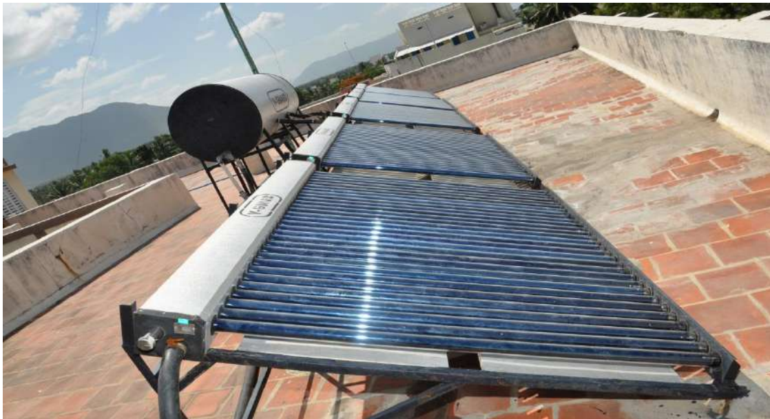
Solar Panels installed in Amalagam Hostel
